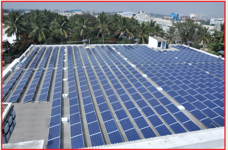
Solar Panel Installations at AUMA India
